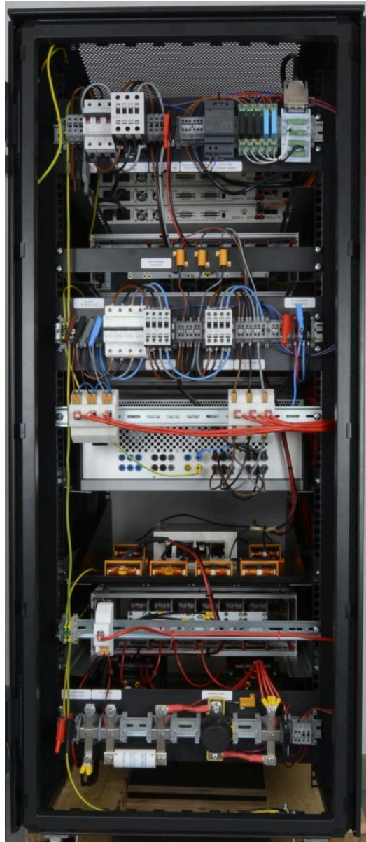
Rear view of the cabinet
